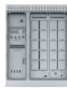
Capacity: 144 kWh Power: 60 kW
